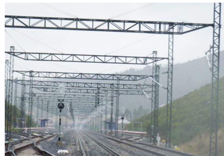
Catenary on the high-speed Atlantic Artery
