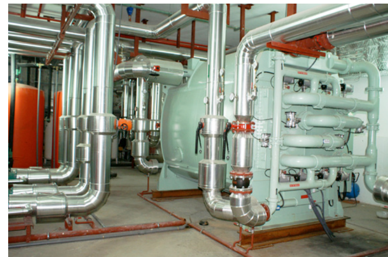
Absorption plant in an athletic complex, Madrid
